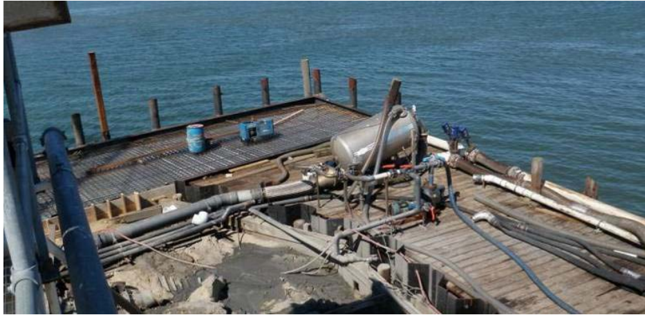
Figure 22. A dockside pump utilized for removing fish from the hold and into the processing facility.
