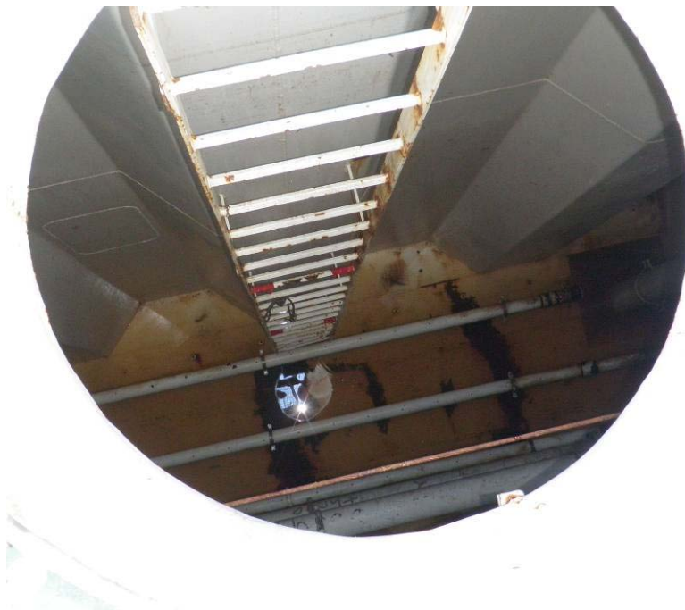
Figure 8. A holding tank, empty
