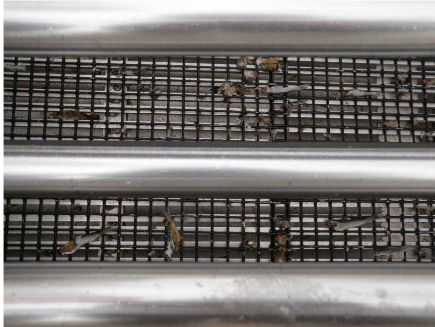
Figure 5. Detail of the lower half of a de-watering box, demonstrating how small marine life and detritus can catch and clog on the mesh
